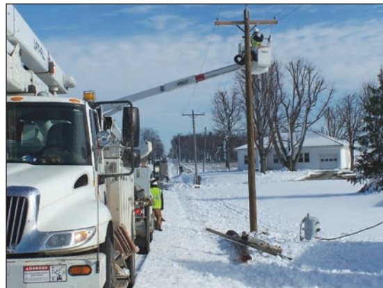
Linemen worked from 6 a.m. to midnight for four days to restore power to all our members.
