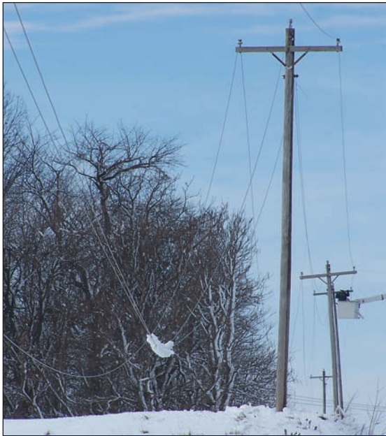
Heavy snow blanketed power lines causing them to sag and eventually break.
