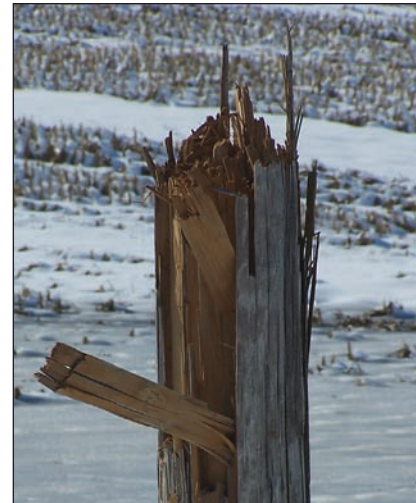
Forty poles were broken and at least 200 miles of power line were damaged during the storm.
