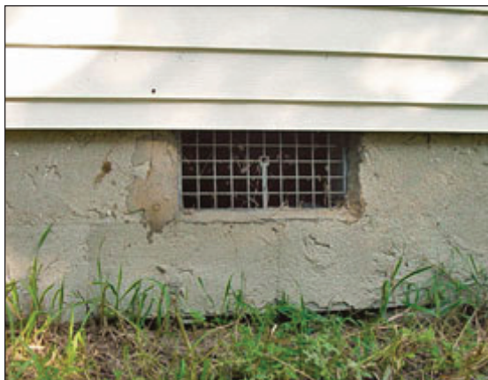
Vented crawlspaces are a great pathway for summer humidity to condense on your floors.
