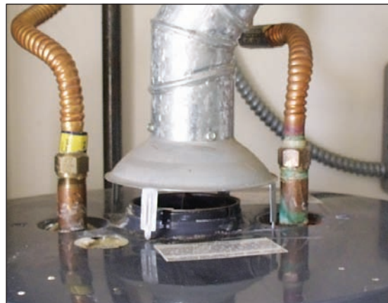
A draft-vented water heater is dangerous.
